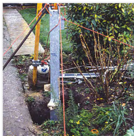
Fig. 6: To keep the mast vertical while the concrete sets, Colin G6MXL tied string around the post in the form of guys to temporary stakes in the ground.
